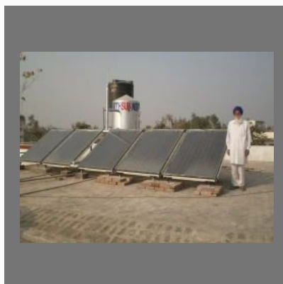
Solar Water Heater System
