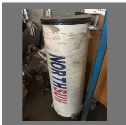
Solar Water Heater Tank
