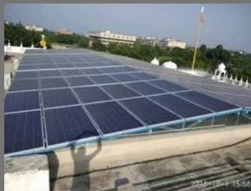
3kW On Grid Solar Power Plant
